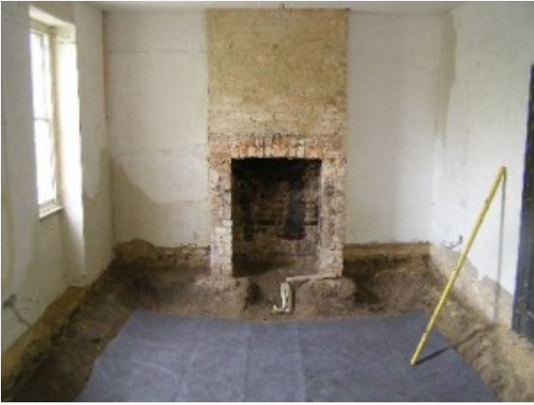
3. After removing 10 tonnes of soil by hand the next job was to lay the geotextile membrane to contain the loosefill
